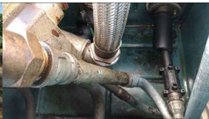
Figura 14 – Interior bomba gasolina
