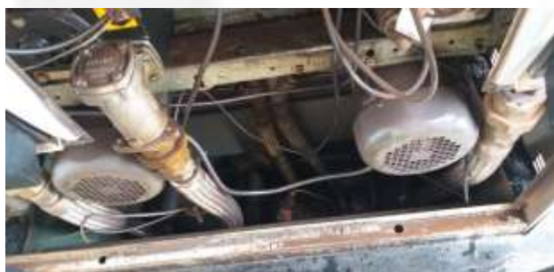
Bombas com sump e check valves
