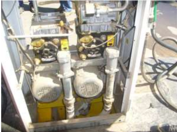
Bombas equipadas com check valves e sump's
